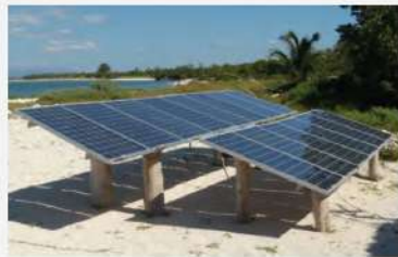
Fig 4 Photovoltaic Solar Panel Array Courtesy of University of St Andrews
