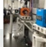
Transport Line LINAC-Booster
